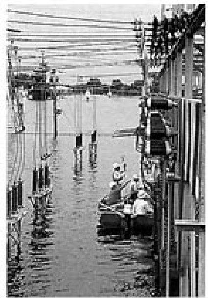
All power companies are exposed to the vagaries of weather. Union Electric Co.'s Huster bulk substation in St. Charles County, Mo., experienced its menacing side when it was flooded four years ago. Photo courtesy of Union Electric Co.
